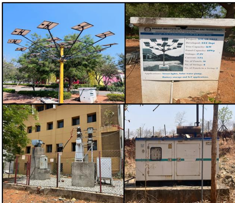
Energy conservation facilities observed in the Campus
